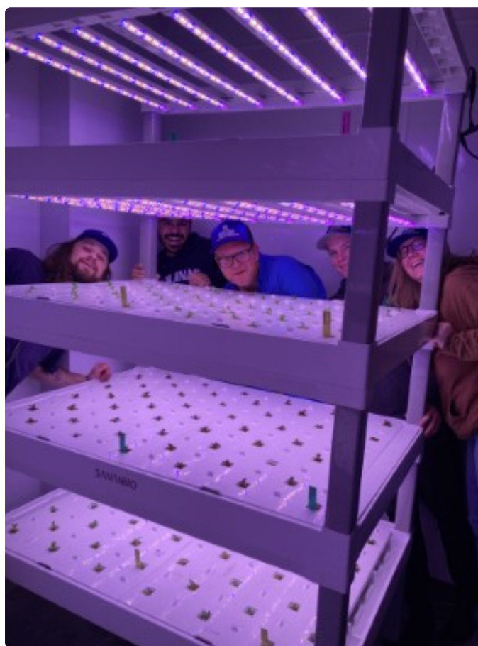
Students in HORT 485R, Horticulture Capstone, install vertical gardens and Dutch Bucket growing systems in the new Winifred school greenhouse and indoor agriculture facility on Oct. 28.
